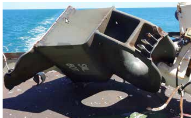
Fairlead pulled from deck. Can be caused by overload or peak load (photo Arie Nijgh, Australia).
